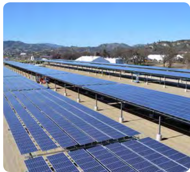
Fort Hunter Liggett Solar Photovoltaic Energy Conservation Investment Program project. (Photo by John R Prettyman)
