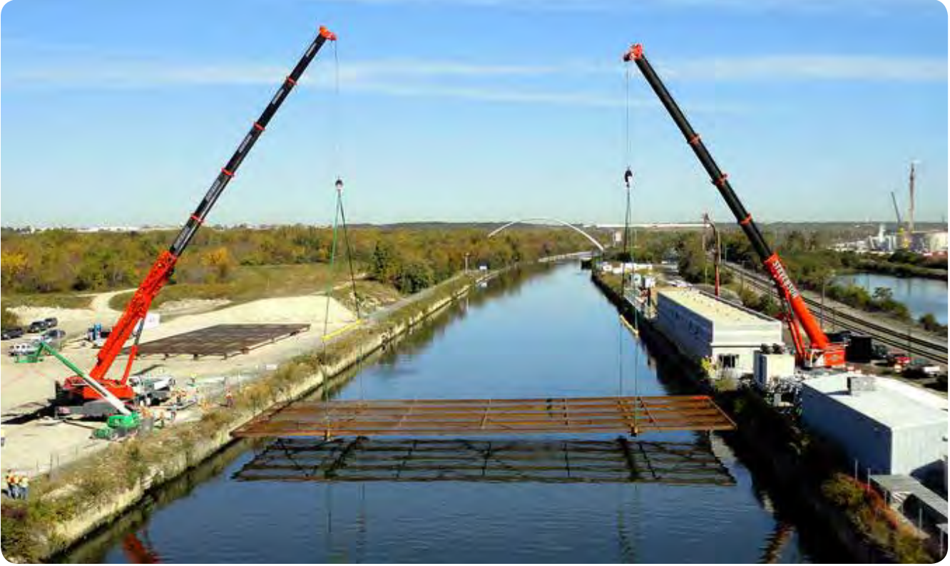
Underwater structures, known as parasitics, being placed into the Chicago Sanitary and Ship Canal by the barriers to the areas designed for fish deterrence. (U.S. Army Photo by Sarah Gross/Released)
