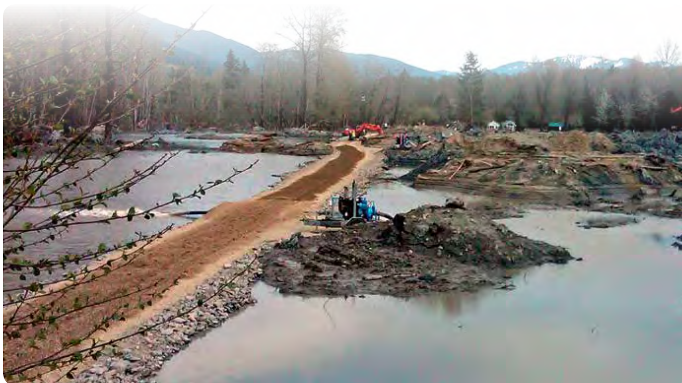
The U.S. Army Corps of Engineers, Seattle District, has nearly completed construction of the temporary berm within the SR530 slide area. (Photo courtesy of U.S. Army Corps of Engineers)
