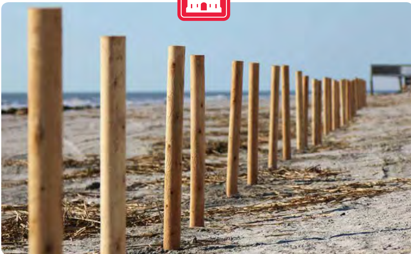
The Charleston District has begun the fencing and grassing project at Folly Beach to build dunes behind the recently completed renourishment project. (Photo by Sara Corbett)
